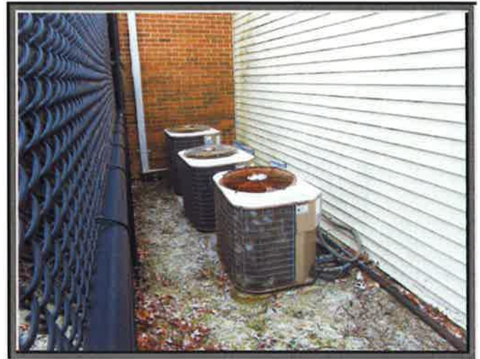
Three HVAC Units
