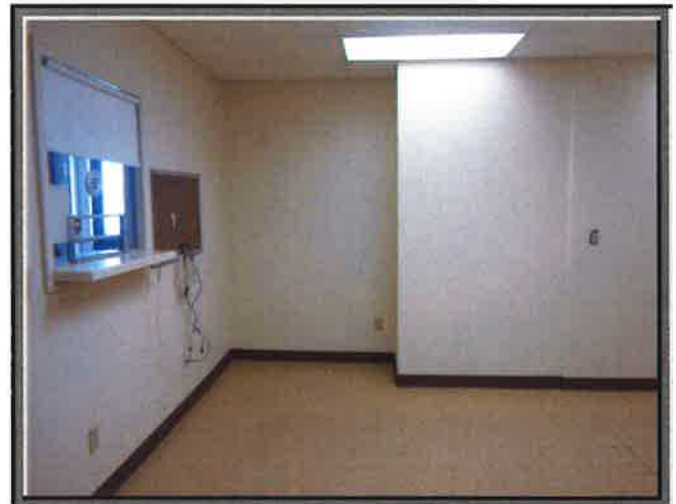
Glass Partition & Office Space
