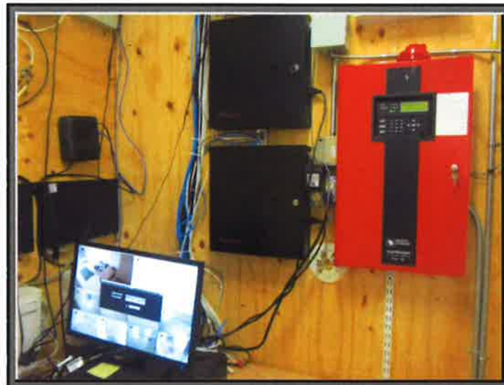
Utility Room - Security & Fire Panel
